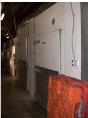
Picture of the shell of our walk in Freezer in need of completion
